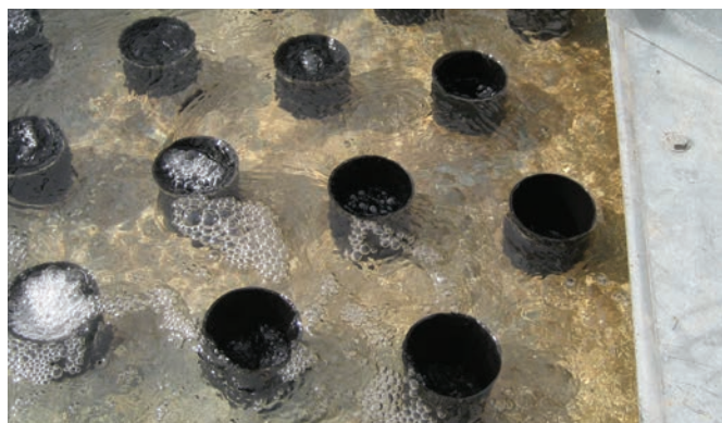
Photo 1: Adding cup extensions to the center pan orifices maximizes contact during low flow at the tower perimeter.
